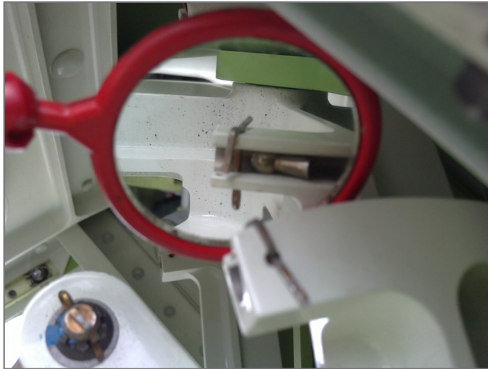
End of the broken cable, held in its housing in the quadrant, seen through a mirror
