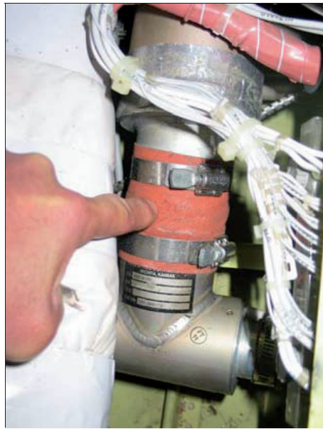
Figure 4: The same equipment after removal of heat insulation
