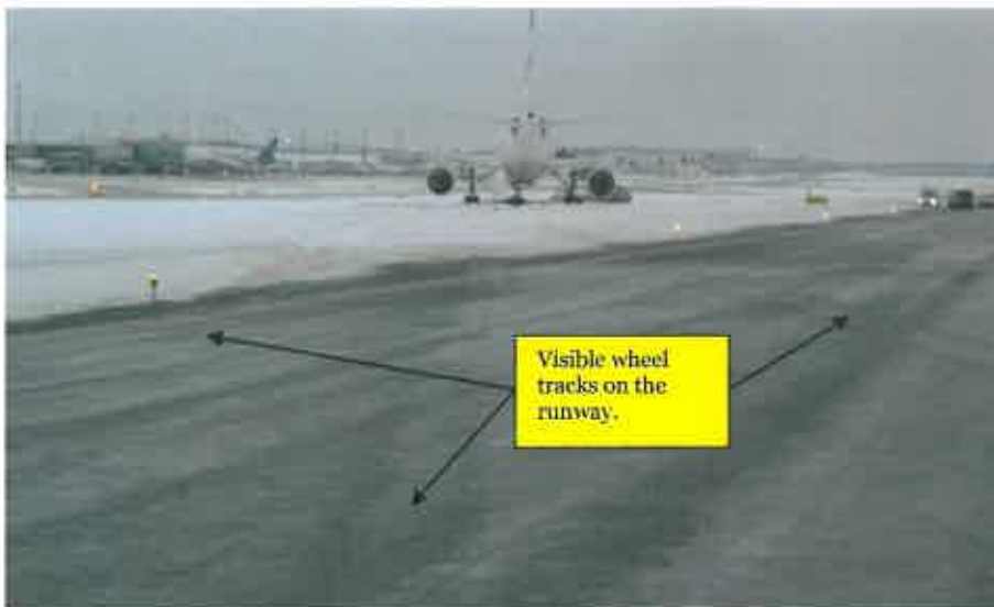
Fig. 35b. Tracks on the contaminated runway surface. Photo: Swedavia.
