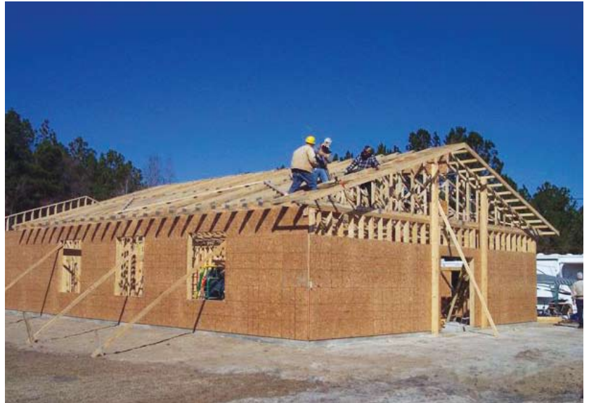
Laborers For Christ, working for Holy Trinity Lutheran Church, Kingsland, Ga., helped expand the church with a 6,290-sq.-ft. addition.
