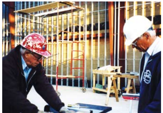
Laborers Ken Wilbur, left, and Norm Hoppmann work on the new family life center for Salem Lutheran Church and School, Springdale, Ark. The facility includes a nearly full-size gym floor, a small kitchen, and a mezzanine to be used primarily as a youth room.
