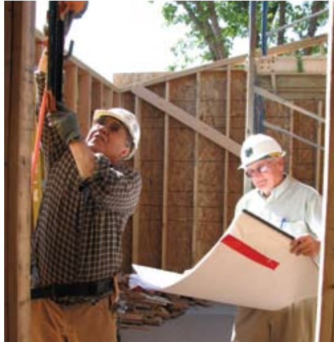
Holy Cross Lutheran Church is participating in the Laborers For Christ program to build a 1,139-square-foot expansion in Atwater, Calif. Laborers Jose Avila and Doug Strohman are among those tackling the project that will give the church a "more welcoming" entrance, a deluxe kitchen, and more accessible restrooms.
