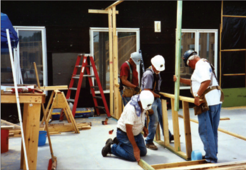
Laborers, working for Peace Lutheran Church, Andover, Kan., erect walls for the 8,200-sq. ft. hall that will replace the double-wide trailer the congregation now uses for fellowship activities.
