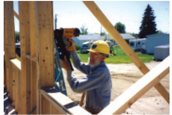
Dale Busse from Akron, Ohio, works atop a ladder at the Sheridan, Wyoming, project site. Busse and his wife, Lucy, former missionaries, have worked with LFC since 1996.
