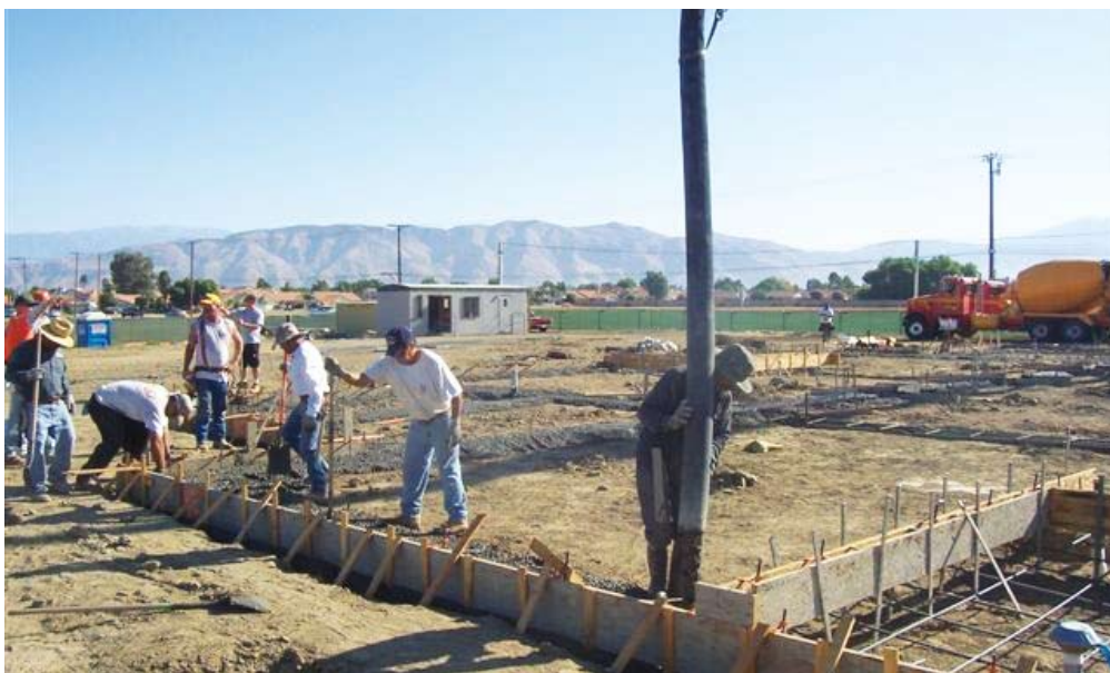
Laborers and volunteers, working for Prince of Peace Lutheran Church, Hemet, Calif., start construction on the 11,400-square-foot family life center that will give the growing congregation more space for ministry and community outreach activities. The building is expected to be complete this
